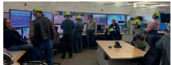
We were also able to view the monitoring and operating systems.
